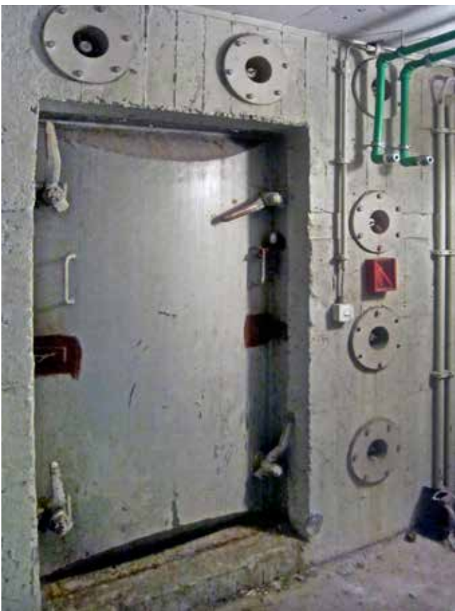
A blast door gave access to the bunkered basement. Photo Günther Schäfer - Alexis Forum
